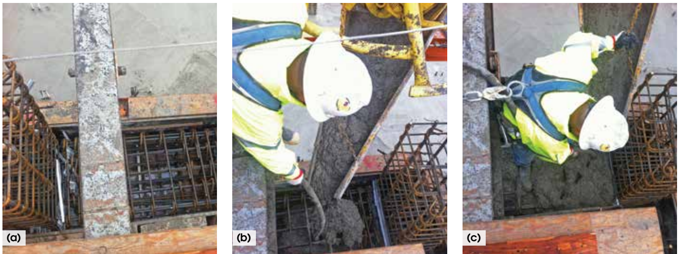
Fig. 2: Construction of a fiber-reinforced concrete link beam in The Martin: (a) reinforcing bars and expanded steel stay-in-place forms are positioned between a column and a wall; (b) a worker consolidates the fiber-reinforced concrete with a spud vibrator as he directs the concrete into the form; and (c) vibration is continued as the concrete is topped off
